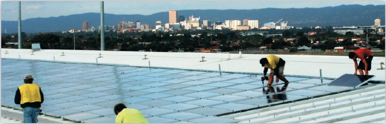
Solar panels on T1 rooftop
